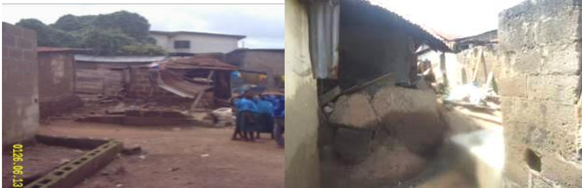
Plate 4: State of building dilapidation in the city core.
