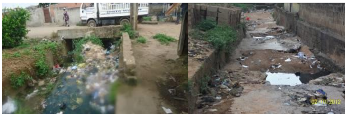
Plate 2: Poor condition of Drainages in the Study Area.
