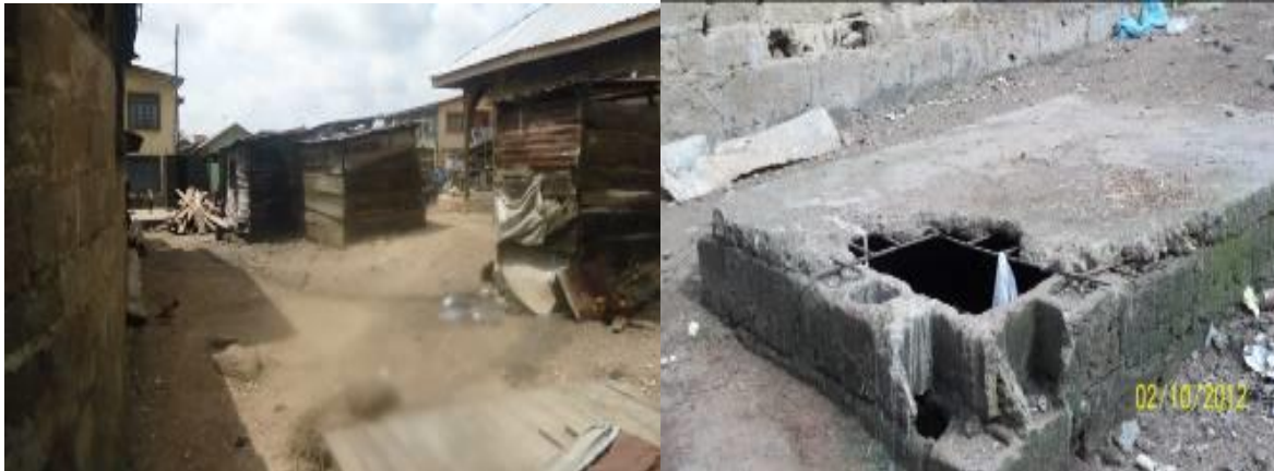
Plate 1: Pit toilets built outdoor and Dilapidated Septic Tank in the Study Area.
